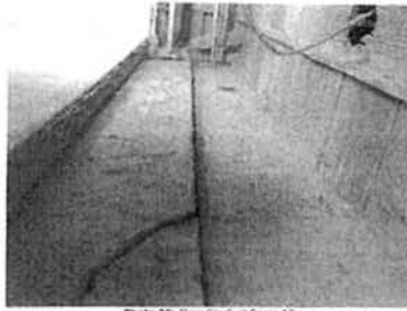
Photo 25: Floor Crack at Room 12
